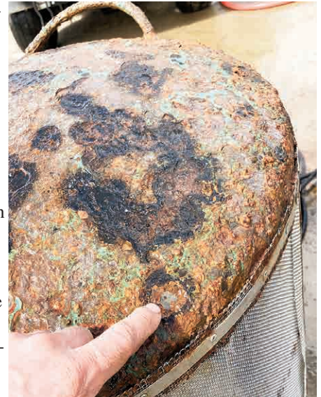
Hole in top of intake screen canister
