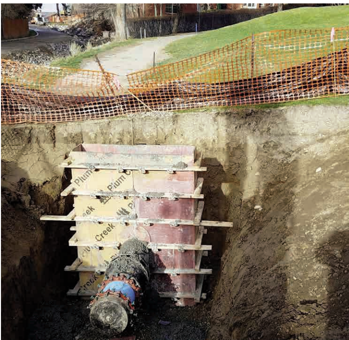
The 18-inch directionally drilled portion with the fitting to transition to 16-inch PVC
